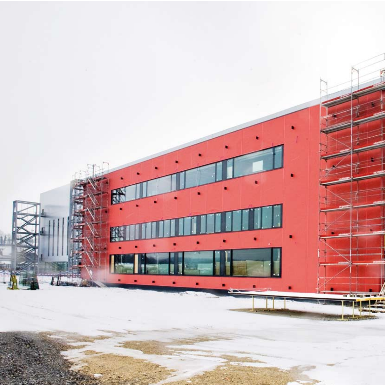
The production and distribution center of Nestlé Nespresso SA in Avenches under construction.
